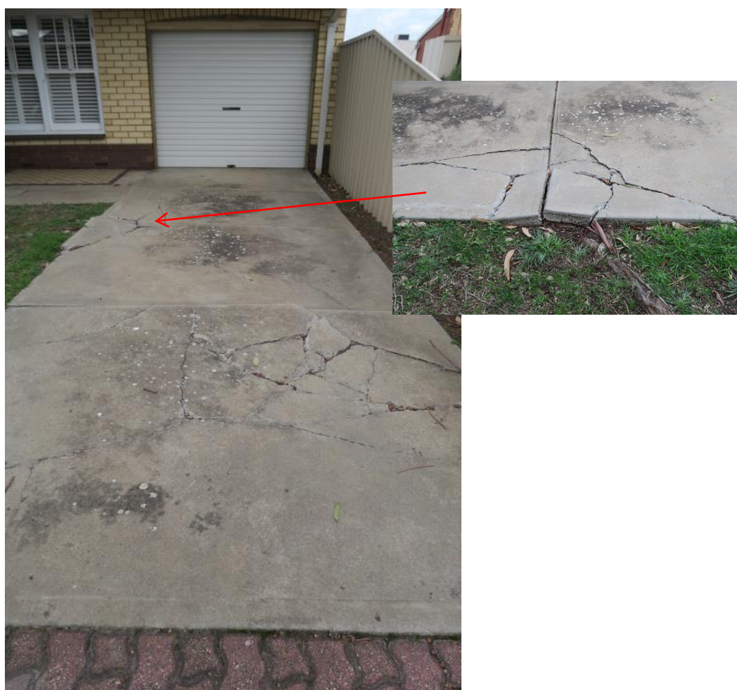
Figure 5. Note damage to concrete driveway.
