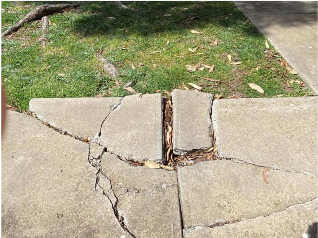
P08 Tree roots in front garden & damaged driveway
