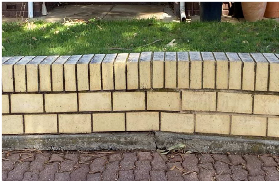
P05 Brick fence - vertical distortion and cracked footing
