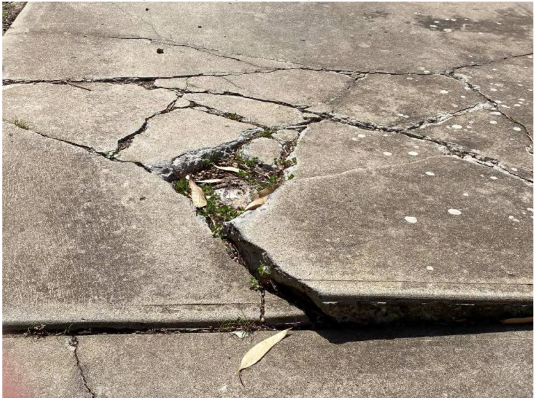
P09 Damaged driveway – tree roots visible
