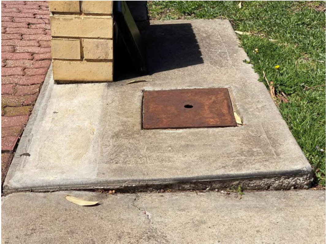
P10 Tilting of concrete pad
