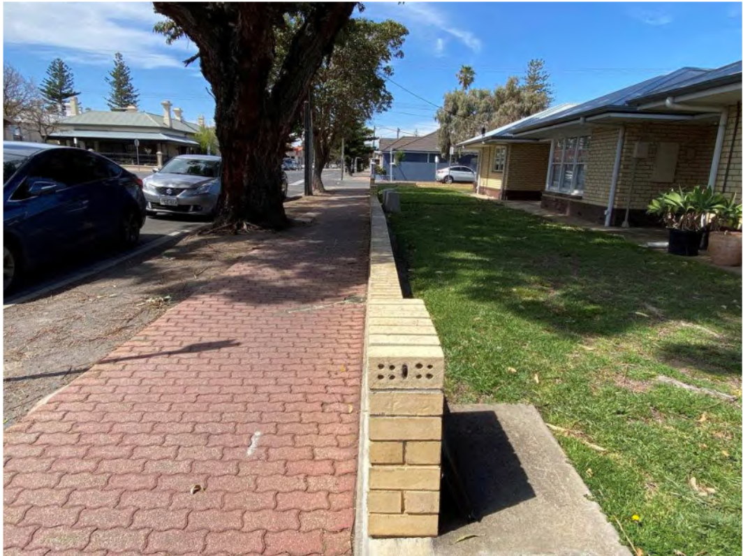
P02 Brick fence - horizontal distortion & tilting
