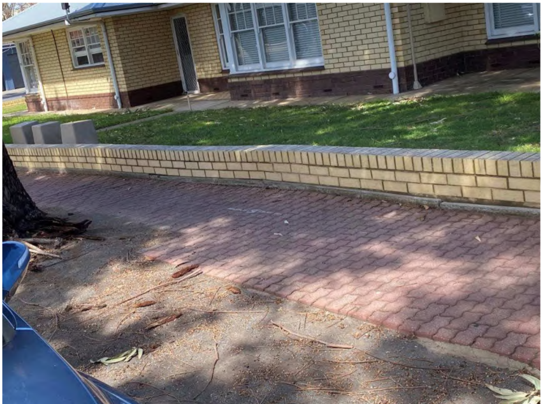
P04 Brick fence - vertical distortion
