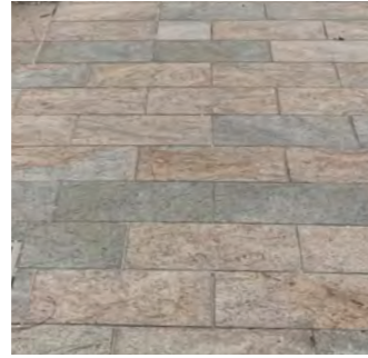
Feature Paving + Crossings - Juperana Granite Urbanstone - Juperana Granite - Stretcherbond with inlay (Feature Paving) and Herringbone (Crossings) - 400 mm x 200 mm x 40 mm
