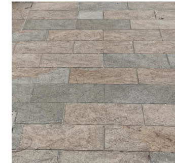
Feature Paving + Crossovers Feature Paving: Urbanstone Juperana Granite - 400 mm x 200 mm in Stretcherbond with inlay
