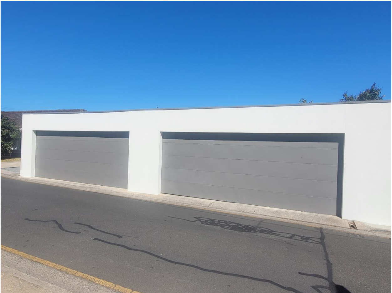
Photo showing the garage doors that will be overshadowed in the morning of the winter solstice
