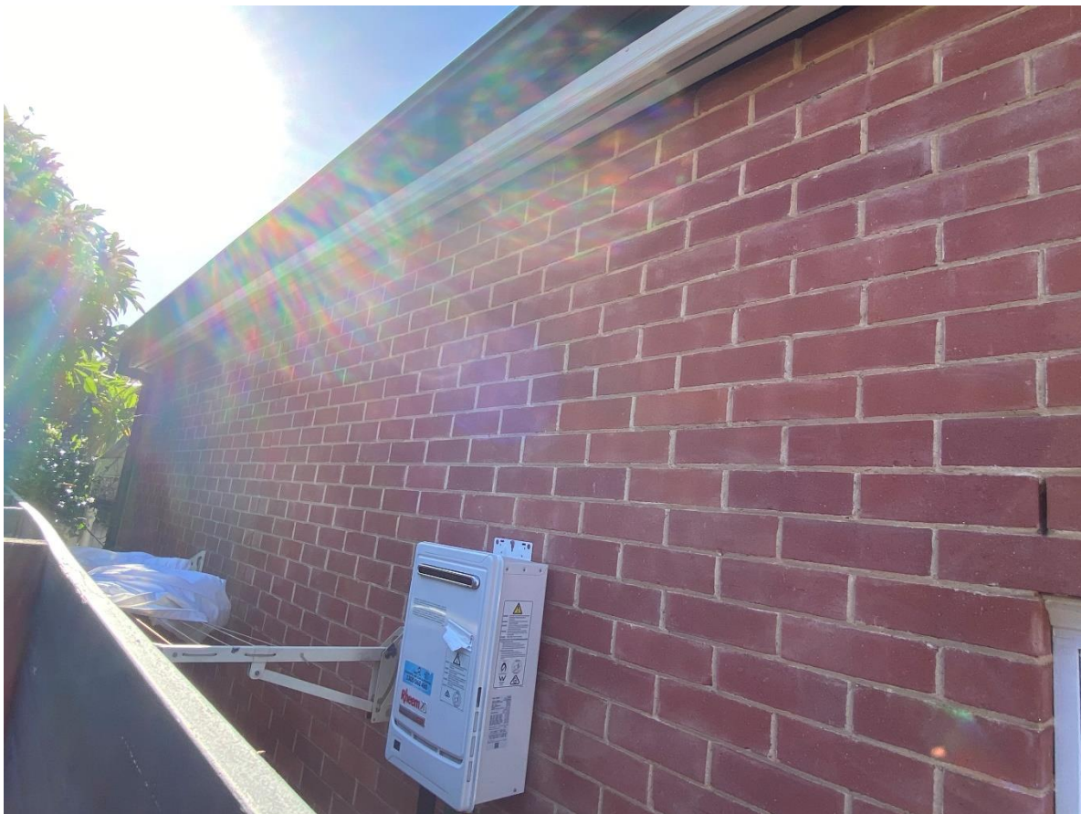
Above: The image of the wall associated with the family/dining room of 16 Gordon Street
